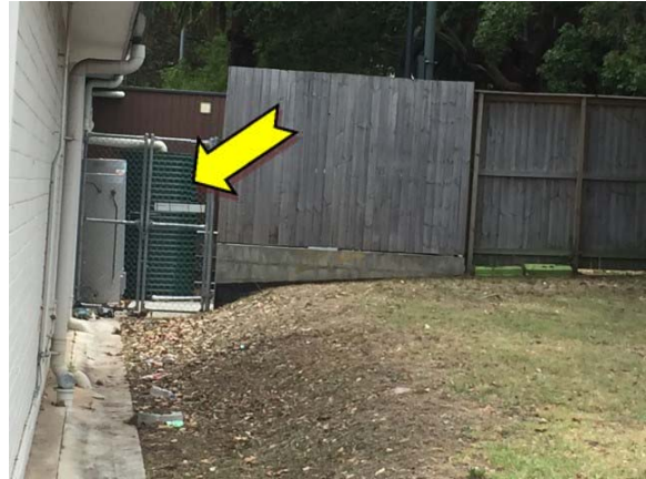
Photo 8. Exterior, north elevation, hot water heater – suspected SMF internal insulation.
