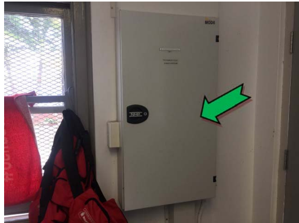
Photo 4. Interior, first aid room, electrical backing board – suspected non asbestos-containing bituminous backing board.
