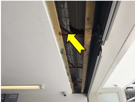
Photo 9. Interior, reception and café, ceiling space – suspected SMF sarking insulation.
