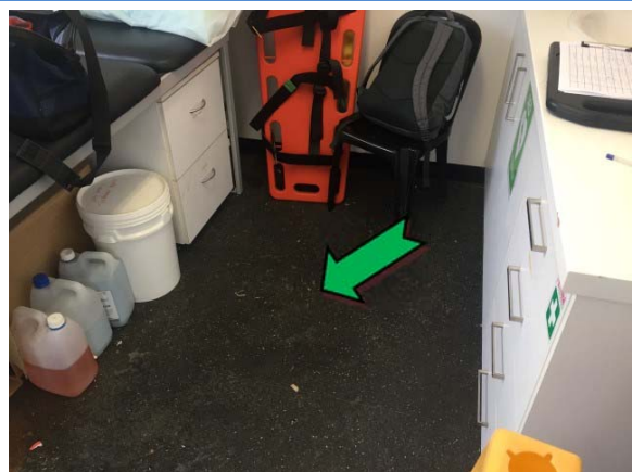
Photo 6. Interior, first aid room, black floor coverings – suspected non asbestos-containing sheet vinyl.
